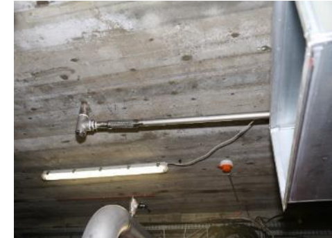
Collector pipe at lowest point of floor
