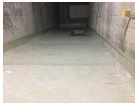
Retention tank 1: 1900 L
