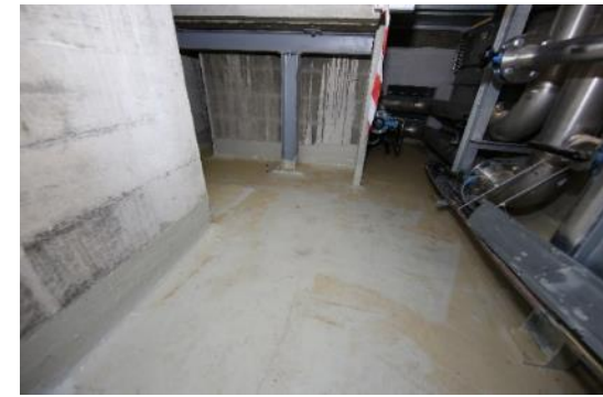
Retention tank 2: 1900 L
